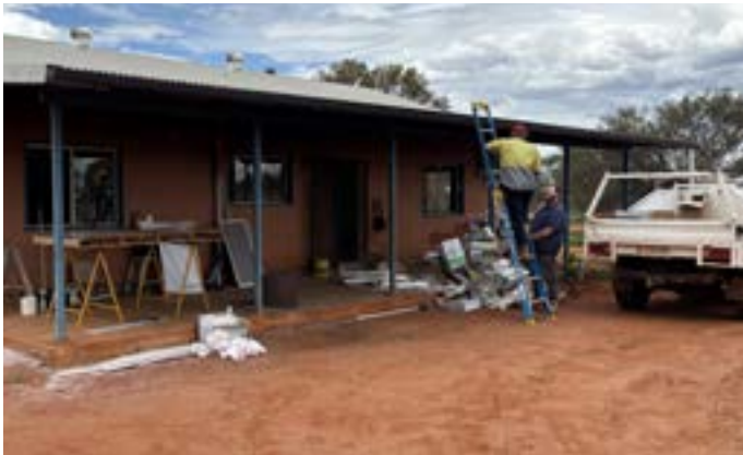
Tywenpe Burt Creek Anpaneye Solar installation Dec 24
